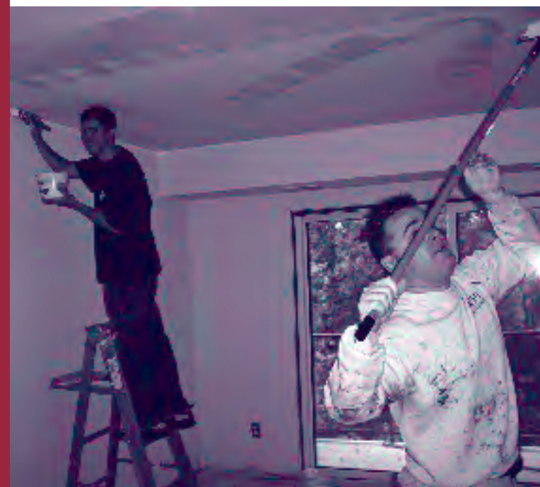
Mount Vernon Kiwanis members help paint an apartment unit for a new Good Shepherd Housing Family.
